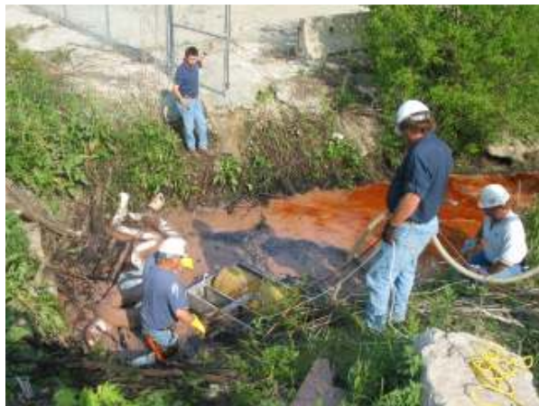
Drum skimming operations 500 gallon waste oil spill, Council Bluffs, Iowa
