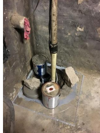
Figure 9-7. Sump More Permanently Sealed with Plexiglass Cover and J-Valve
