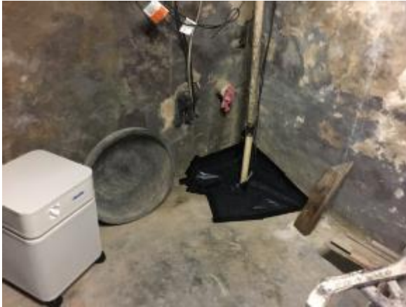
Figure 9-6. Sump Temporarily Sealed with Plastic and Tape
