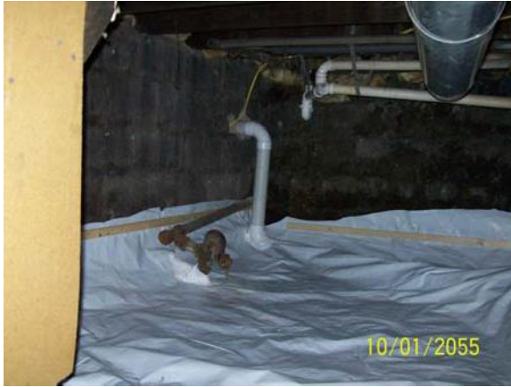
Figure 9-21. Piping Beneath Membrane
