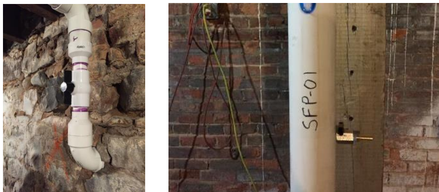
Figure 9-14. Installations of Flow Adjustment Valves (Left) and Sampling Ports (Right) on Piping
