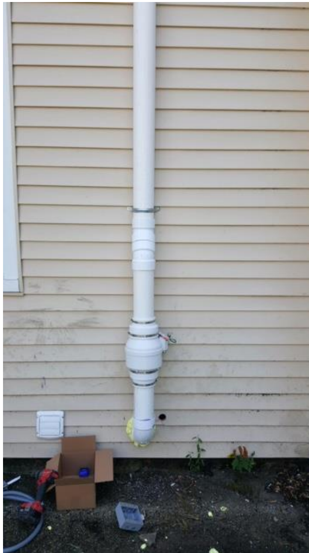
Figure 9-15. SSDS Extraction Fan
