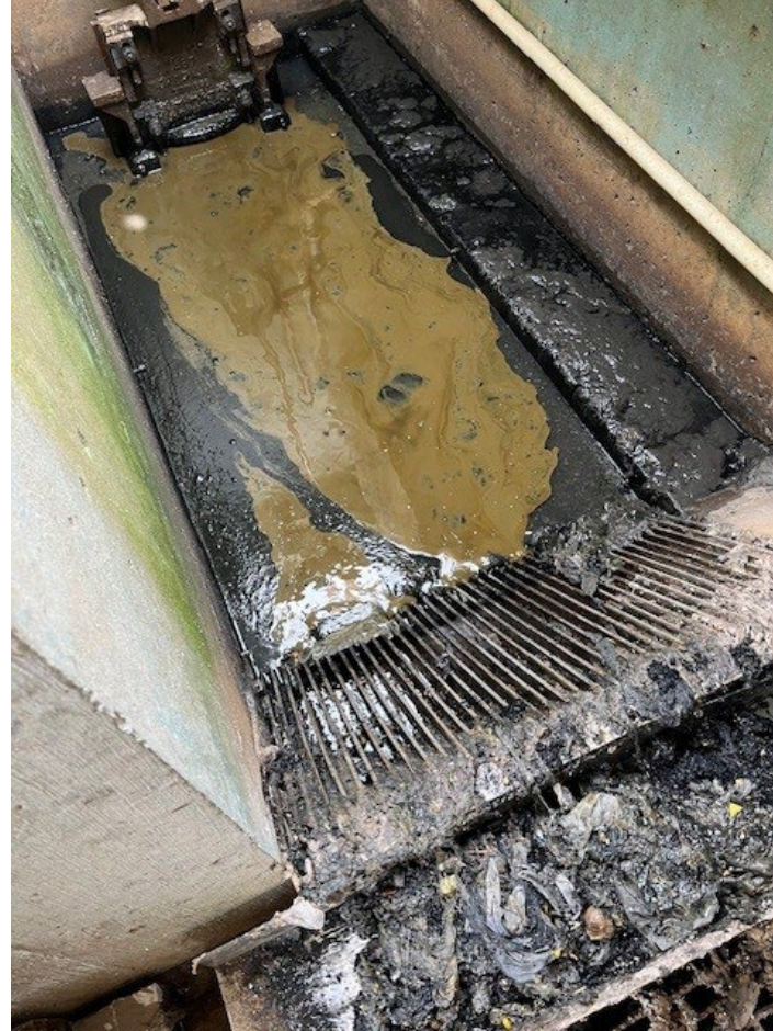
Waterloo WWTP inflow. Oil entering WWTP.
