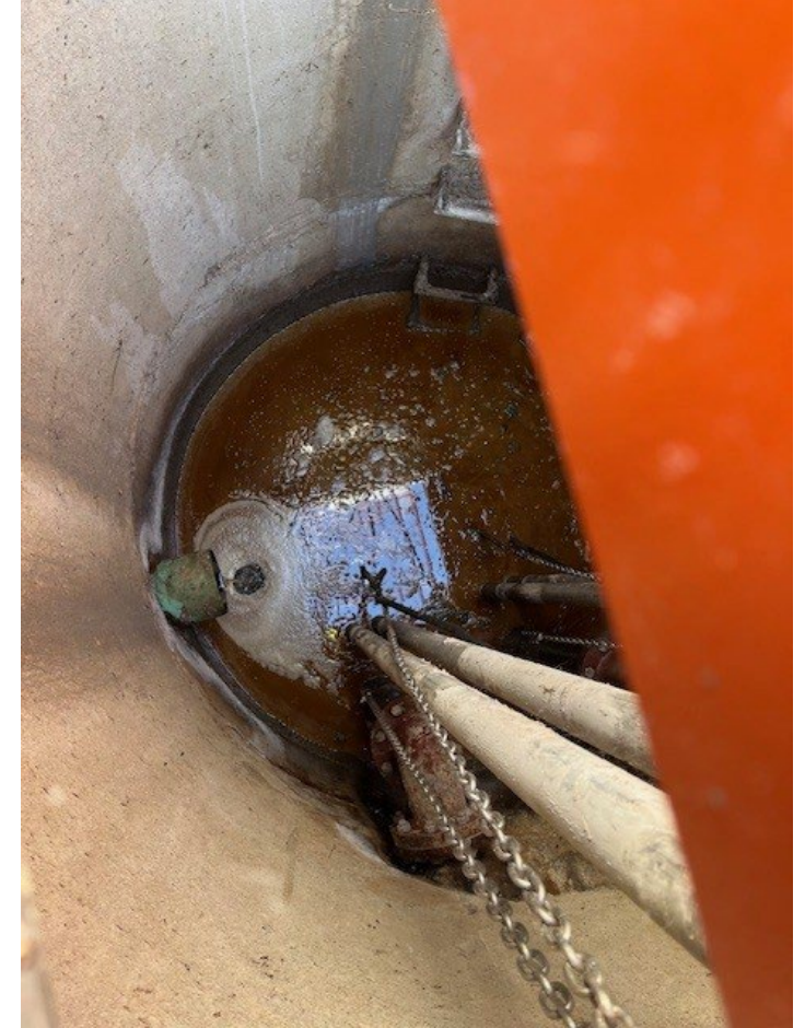
Waterloo lift station. Oil present in structure.
